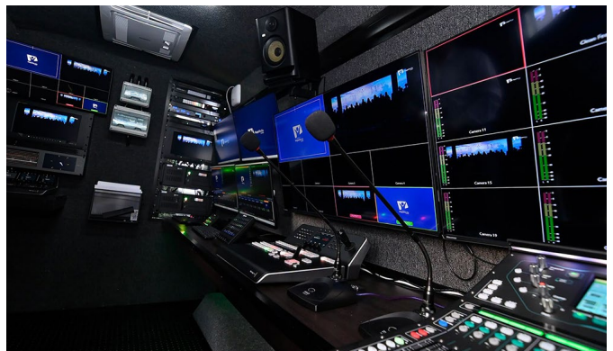
The interior of the mobile production truck features specialized equipment for television production, live broadcasting, streaming, and digital content distribution. [Photo: Chiapas Mexican Union]
