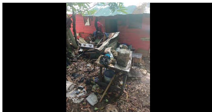
The dilapidated Westmoreland dwelling shared by brother Kennel George Cornwall and his cousin Devellie Lonely prior to intervention by the Cave Church. :: Photo credit: Contributed
