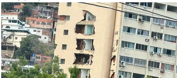
Many apartment buildings in Caracas were left uninhabitable after twin earthquakes struck north-central Venezuela on June 24, causing widespread structural damage. [Photo: Central Venezuela Conference Facebook]
